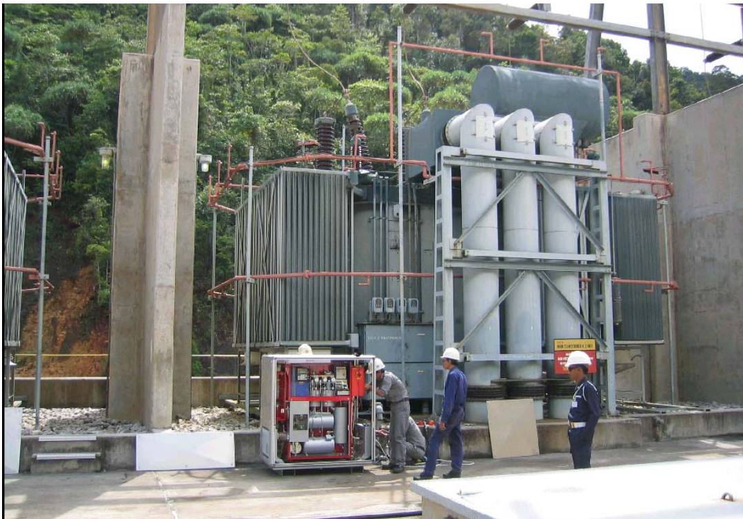
Germany: 250 MVA Transformer
